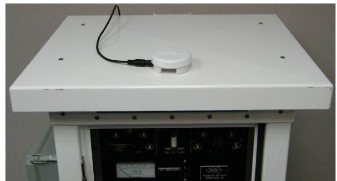
Mounted on rectifier cabinet
